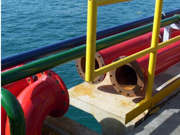
Fire Water Pipe Expansion Joint
